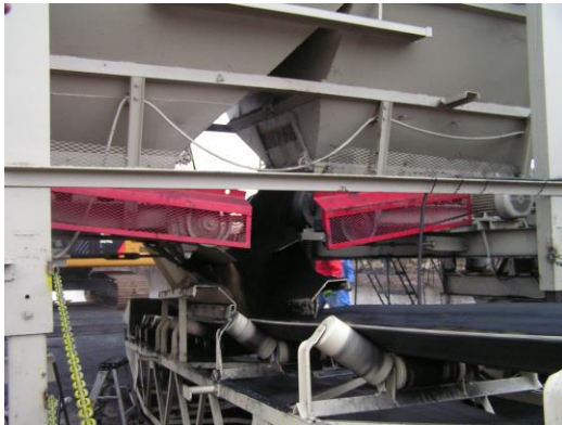
Dual Hopper Sand/AquaGate+PAC Mixing
