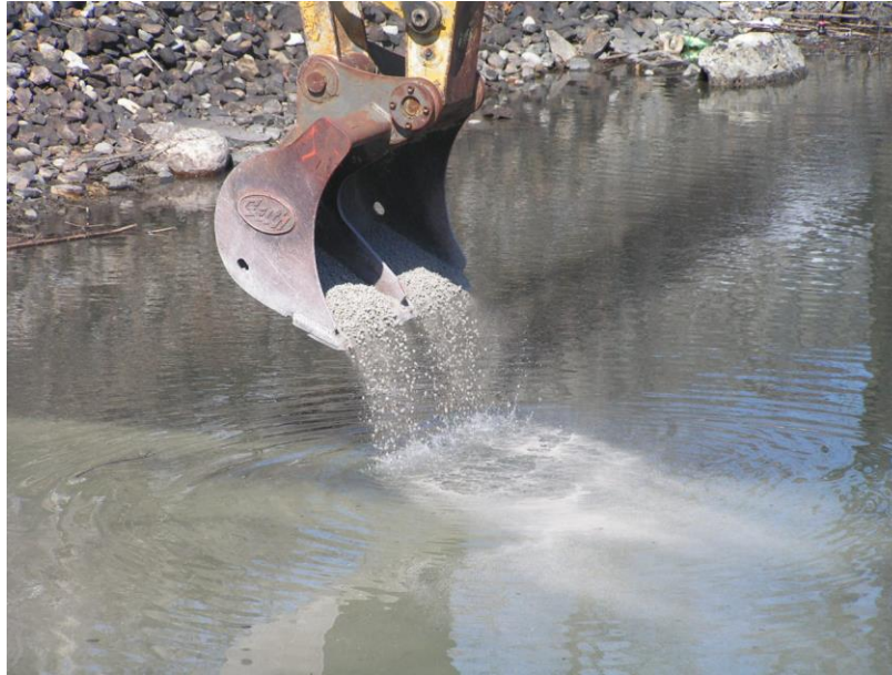
Placement of AquaBlok+ORGANOCLAY product through the water for treatment/adsorption of petroleum-based hydrocarbon contaminants
